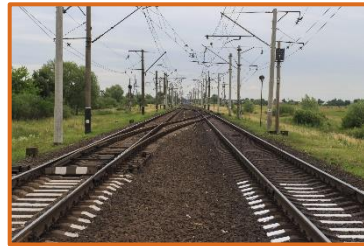
Ile de France railway electrification
